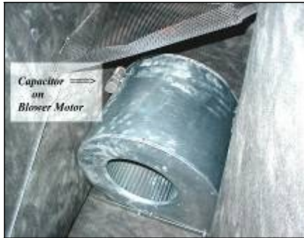
Prohibited: Capacitor on blower fan motor
