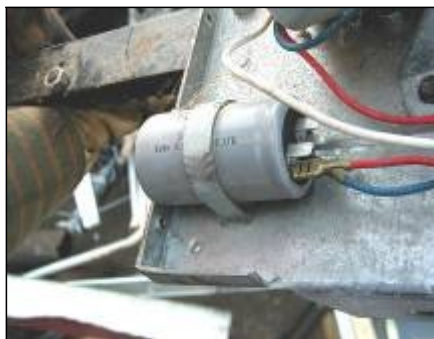
Prohibited: Capacitor in repaired fridge
