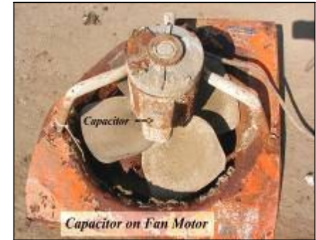
Prohibited: Capacitor on fan motor
