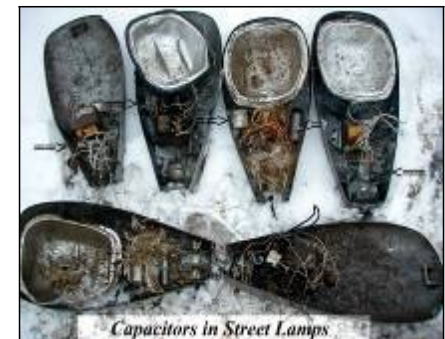
Prohibited: Capacitor in street lamps
