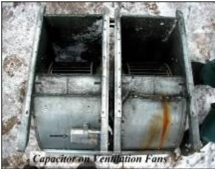
Prohibited: Capacitor on ventilation fan motor
