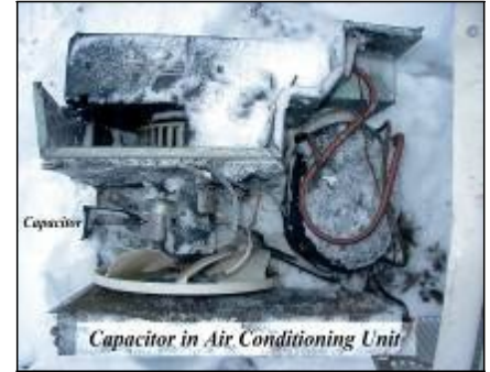
Prohibited: Capacitor in air conditioning unit
