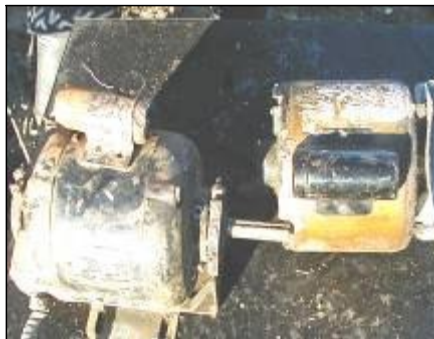
Prohibited: Capacitor in AC motors
