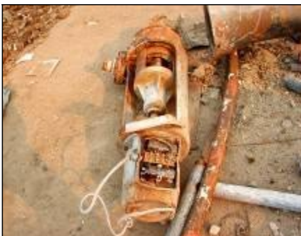
Prohibited: Capacitor in pump motor
