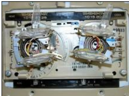
Prohibited: Mercury switches in a thermostat
