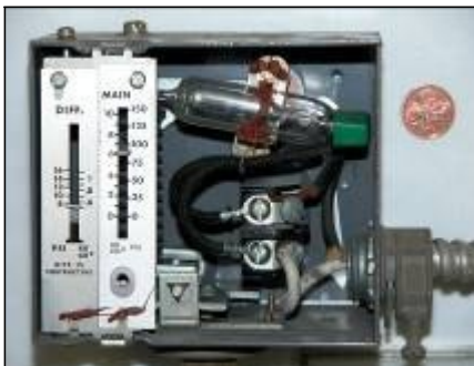
Prohibited: Mercury in pressure and temperature gauges
