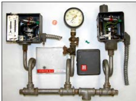
Prohibited: Mercury in pressure and temperature gauges
