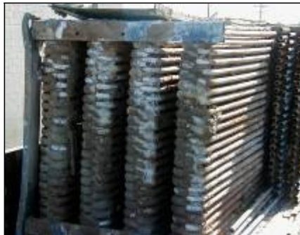
Prohibited: Heat exchanger with deposit/scale
