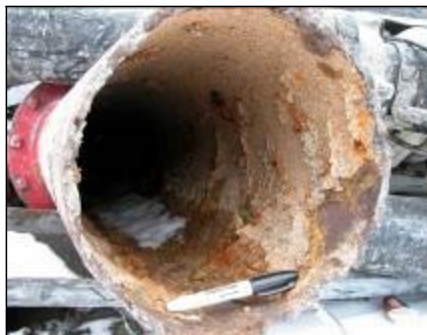
Prohibited: Pipe with radioactive deposit/scale
