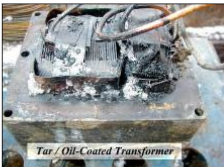
Prohibited: Tar-coated transformer
