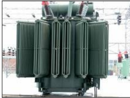
Prohibited: Transformer & components
