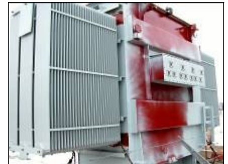
Prohibited: Transformer & components
