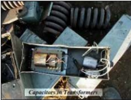
Prohibited: Capacitors in transformer
