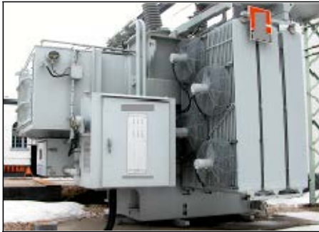
Prohibited: Transformer & components
