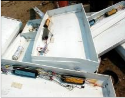
Prohibited: Ballasts on fluorescent light fixtures
