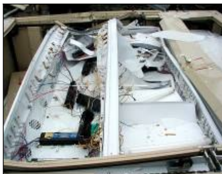
Prohibited: Ballasts on light fixtures in fixture x-ray film reader
