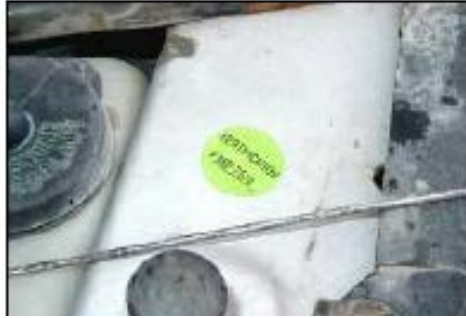
Prohibited: Air-conditioning system containing CFC
